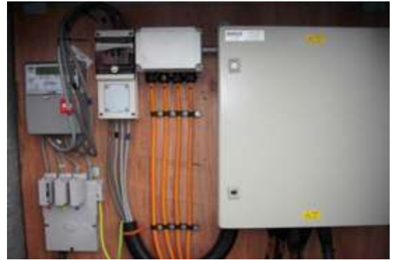
Column Impact Detector Cables – Looped in each Column via Tilt Switch
