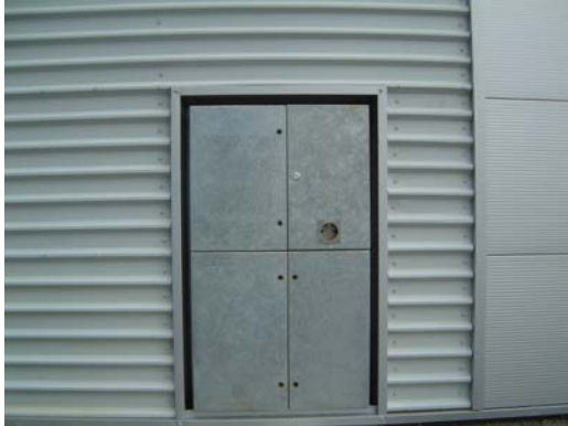
Outdoor Metering Enclosure installed in an industrial premises
